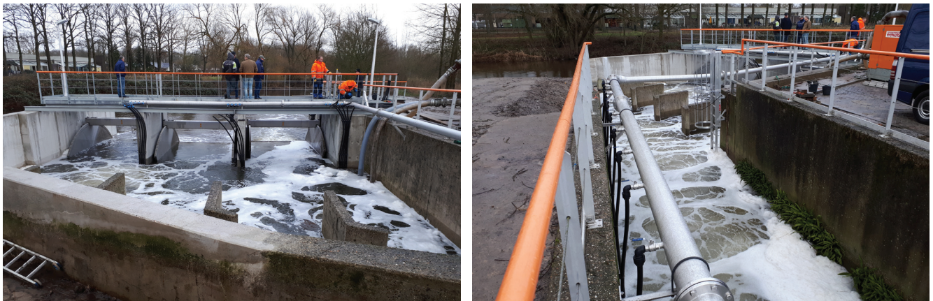
FIGURE 7. The aeration channel of the Eindhoven Wastewater Treatment Plant in full operation as it improves the oxygen quality of the effluent before reentering the Dommel. Left: View of the adjustable dam at the outlet of the aeration channel. Right: View of the aeration channel from the inlet.
