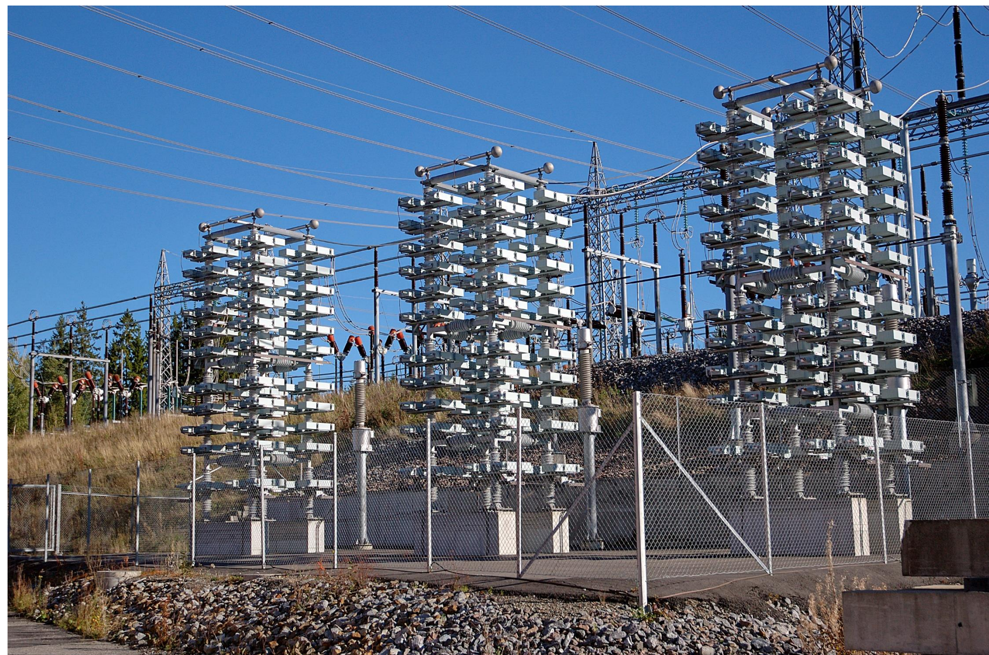
Figure 1. An ABB shunt capacitor bank.
